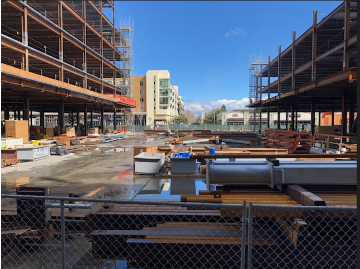
Future Francis Street between the West and East commercial office buildings connecting the new Vargas Street with West Washington Avenue.
